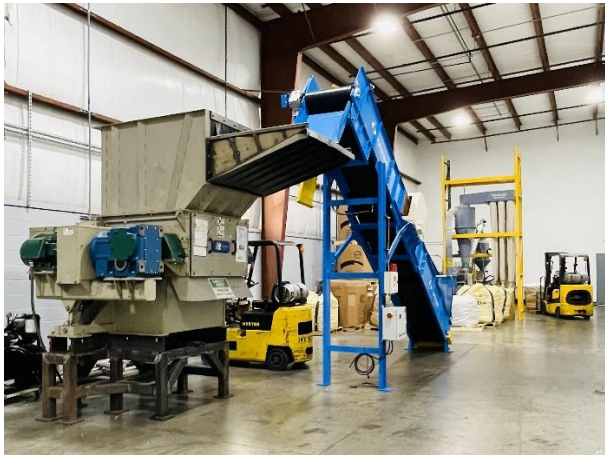
PHOTO: Shredding Machine at Polymer Resources Rochester, N.Y., Facility
